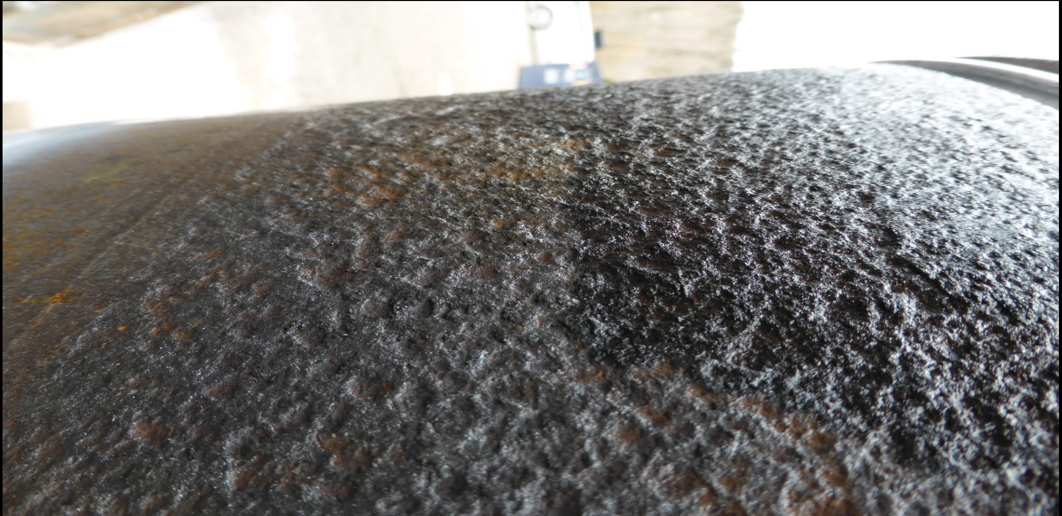
Figure 8: CB Corrosion Sample
