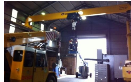
10T overhead crane with Technomagnet plate lifter
