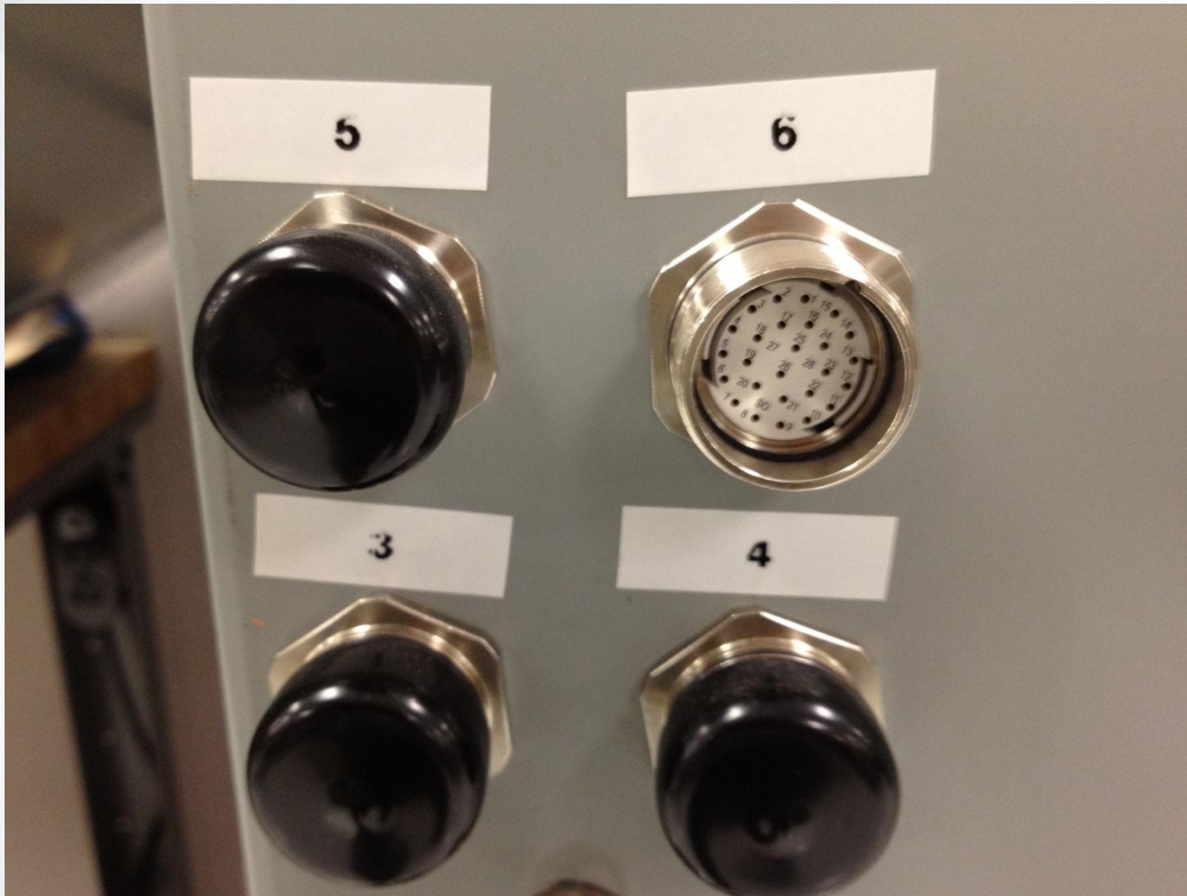
Cable Connectors on Cabinet
